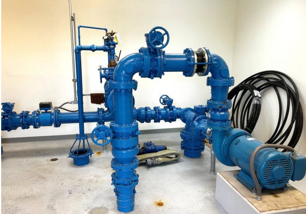
Figure 9 –Booster Pump Station Piping
