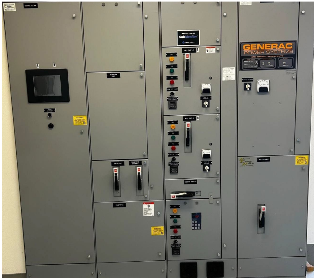
Figure 8 – Booster Pump Station Control Panel
